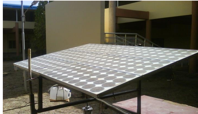
Fig. 1 Six PV panel of each 36 watt connected parallel
